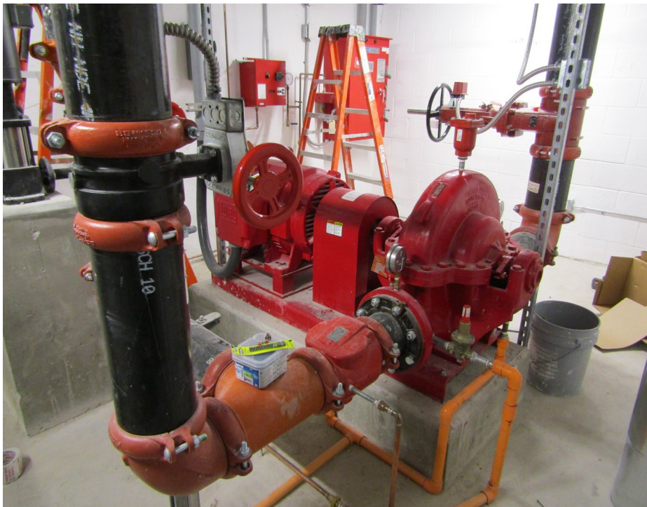
Photo 16 – View of fire pump.
