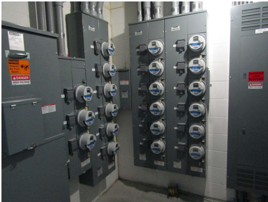
Photo 18 – View of typical meter center in electrical room.
