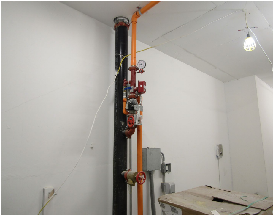
Photo 12 – View of fire safety system.
