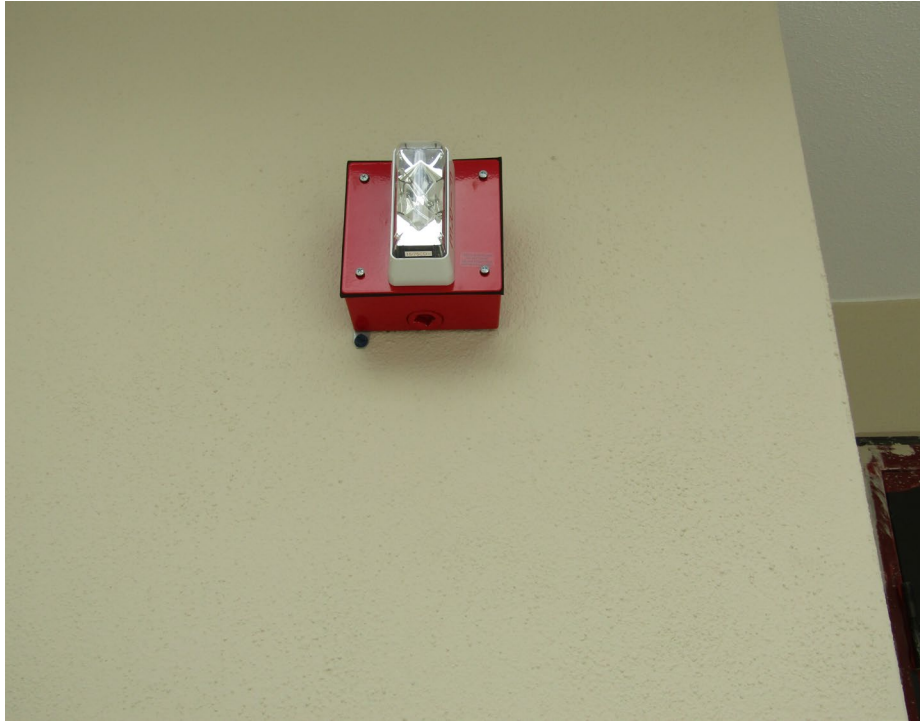
Photo 11 – View of typical fire alert throughout the building.
