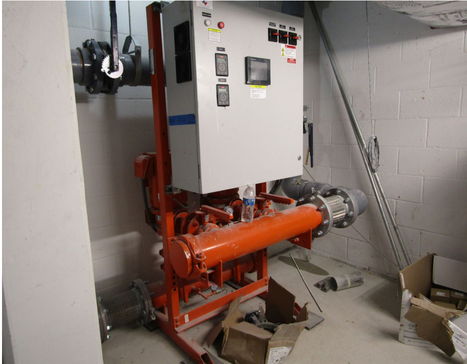
Photo 15 – View of domestic water pump.
