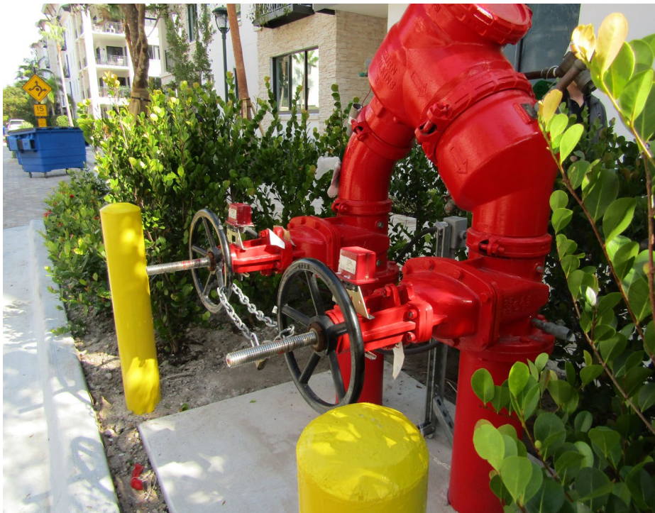
Photo 14 – View of fire sprinkler backflow preventer.
