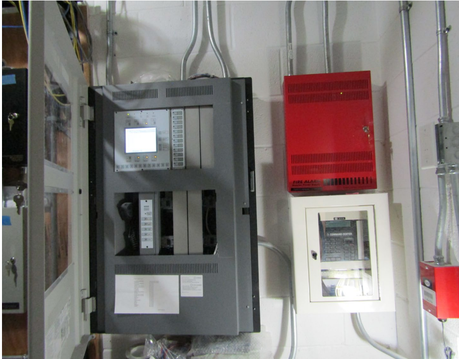
Photo 17 – View of FACP in electrical room.
